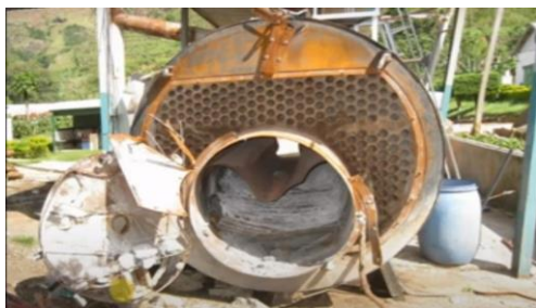
Fig. 7: Front view of the exploded boiler at Demodara tea factory [9]
