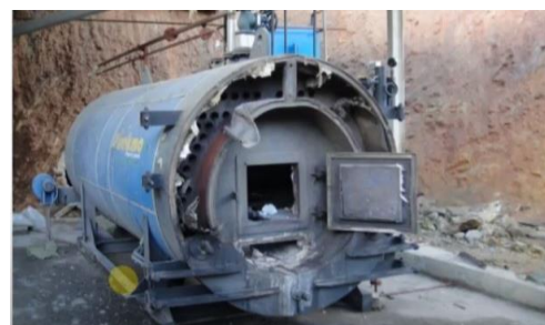
Fig. 6: Exploded boiler at Galle tea factory [2]
