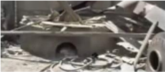
Fig. 2: Foundation of the exploded boiler from the Lanka Rice Mill [9]
