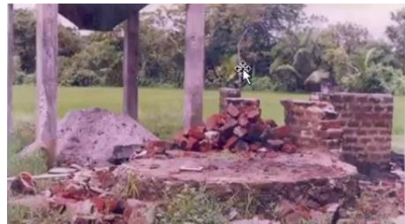
Fig. 4: The collapsed boiler foundation at the Shantha Rice Mill [2]
