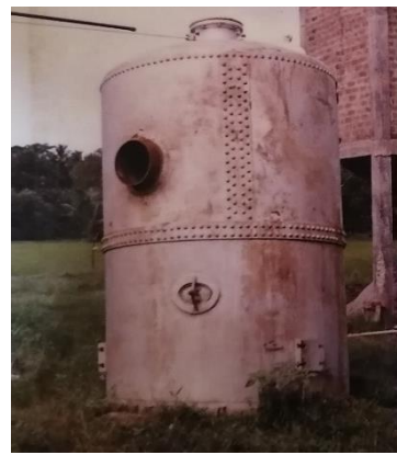
Fig. 3: The Boiler in the Shantha Rice Mill related to accident [9]
