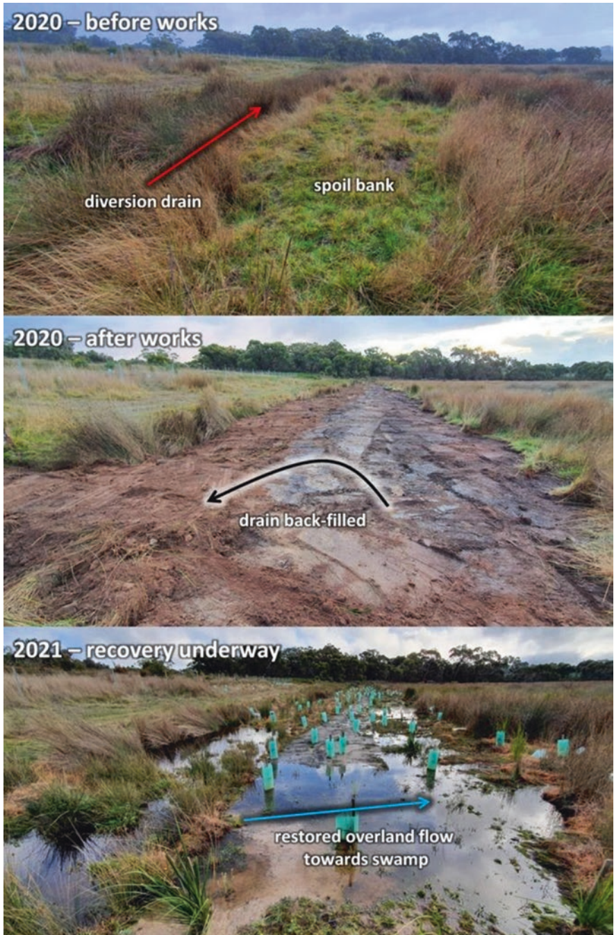
Fig. 6.3 Looking west down a section of the diversion drain at the top of Glenshera Swamp, shown here before and after back-filling in 2020, and again in 2021, showing how the area is re-saturated, restoring flows to the swamp and also being actively revegetated with wetland species
