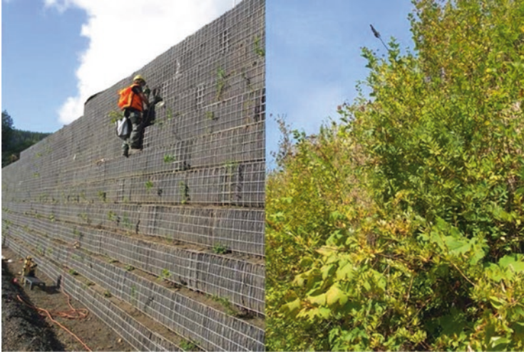
Fig. 9.22 Stepped mechanically stabilized earth wall containing seed-impregnated biodegradable fiber and planted with native shrubs in 2016 and revegetated wall in 2021. (Photo credits Lee Riley)
