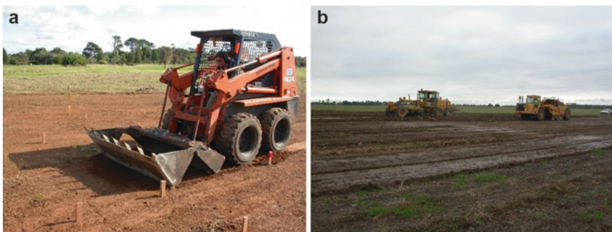
Fig. 2.8 Topsoil manipulation. (a) small-scale excavator ( Left ); (b) large-scale grader and scraper ( Right )
